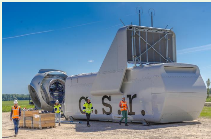
48 new wind turbines a.s.r. invests in wind turbines and solar panels to contribute to the energy transition. The wind turbines, together with a solar park, generate energy for more than 200,000 households
